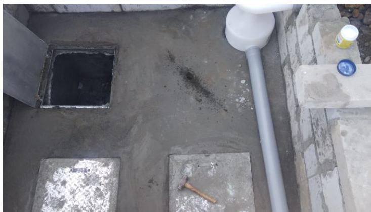
Bio-chamber top view with Aquatron® and inspection manholes
